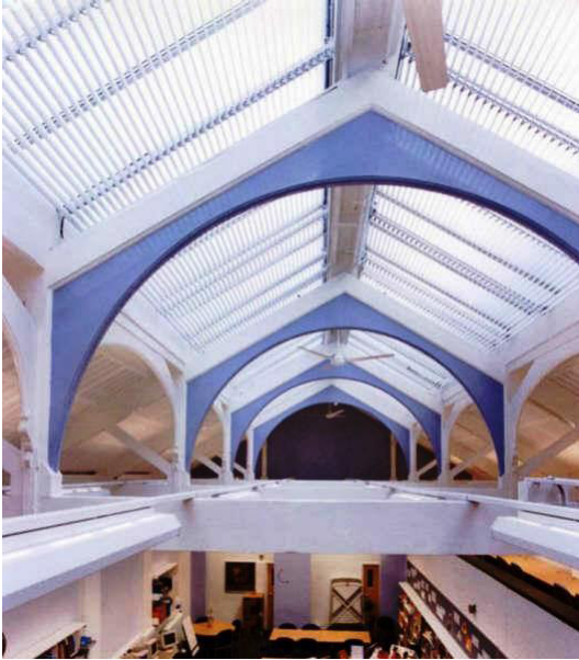
Internal T50 fitted in library
